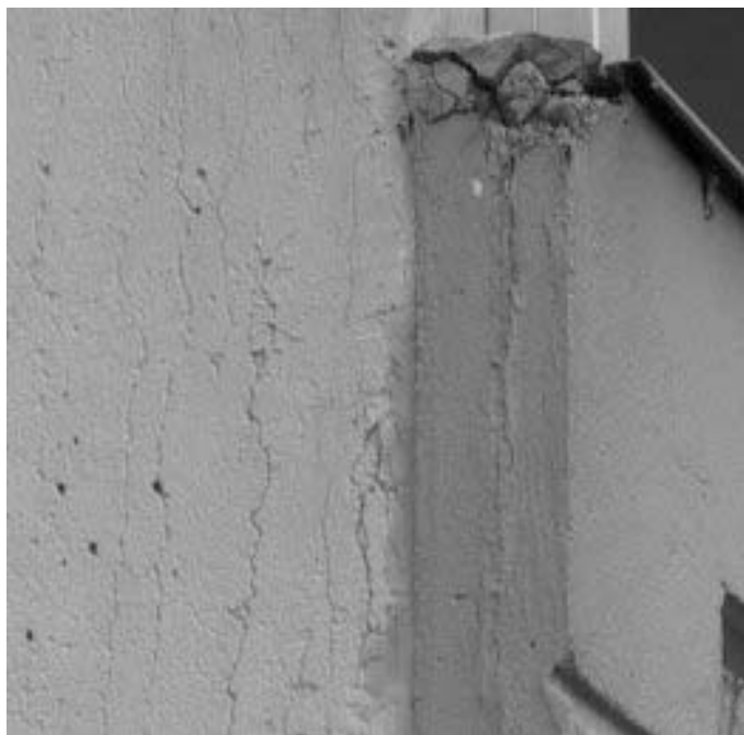
Figure 2. In this case water has exposed the structure to freeze-thaw action. Thus the structure has disintegrated.
