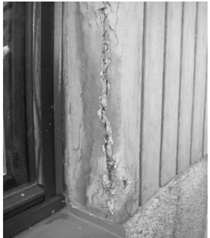
Figure 1. Damage caused by reinforcement corrosion in the window frame
